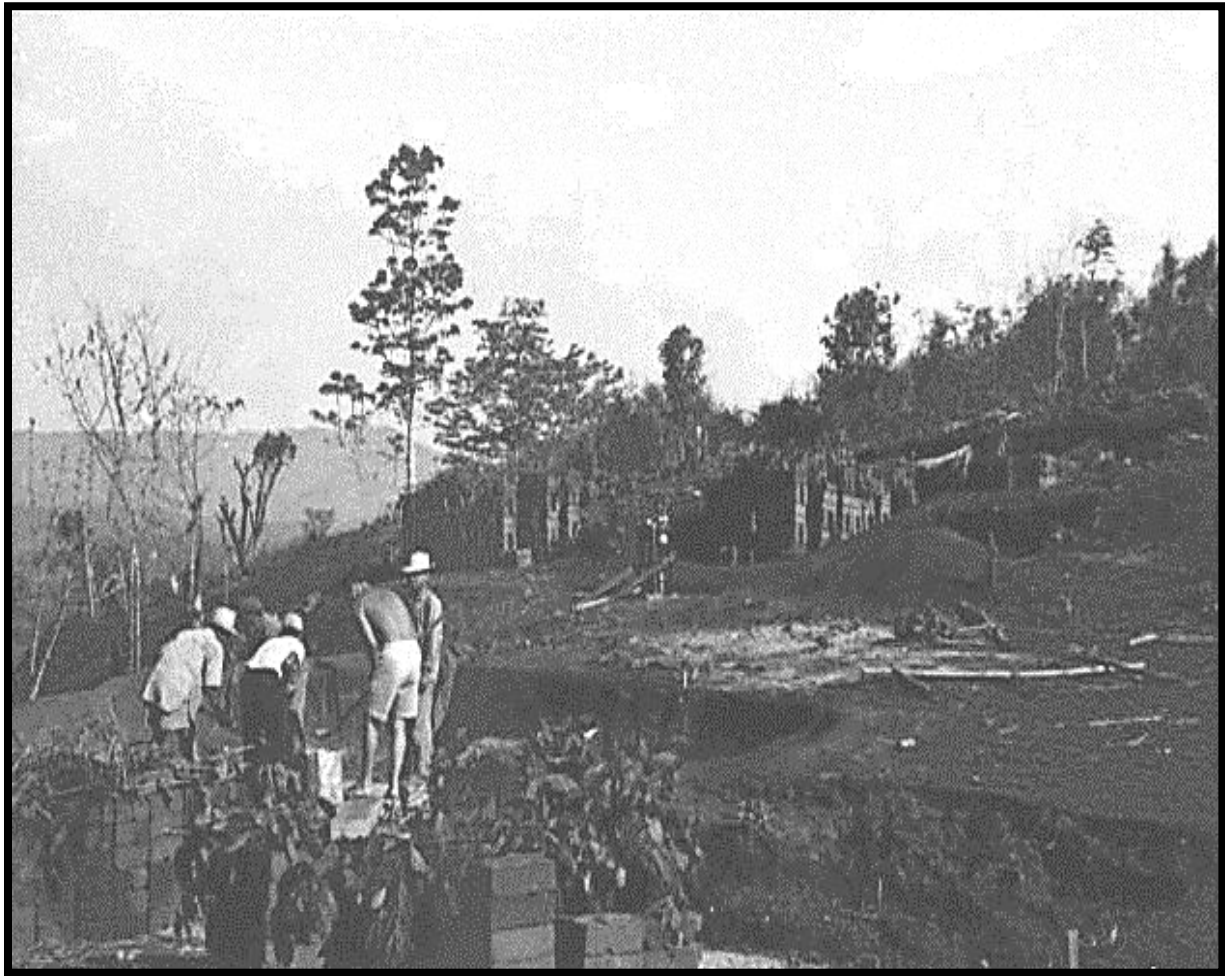
Commencement of the mud block house project at Ban Houei Sai, Laos, site May 1963.
